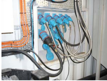
Figure 17 – Electrical connections between modules.
